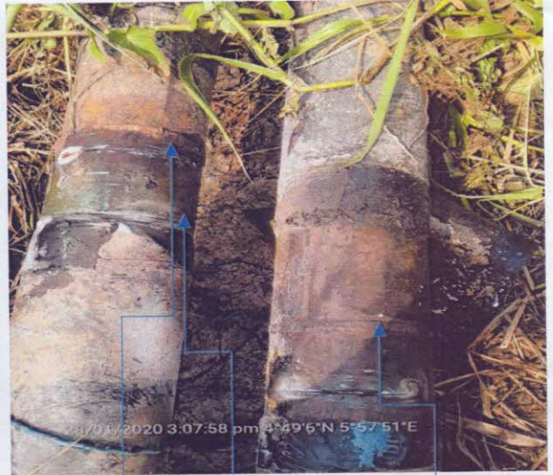
THREE HACKSAW CUTS ON THE FLOWLINE
